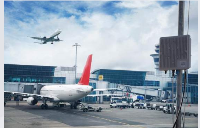
MS27102A mounted on pole monitors airport frequencies for unwanted signals
